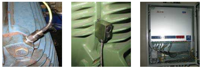
Range of SKF sensors monitoring defined points and SKF IMx online surveillance system
